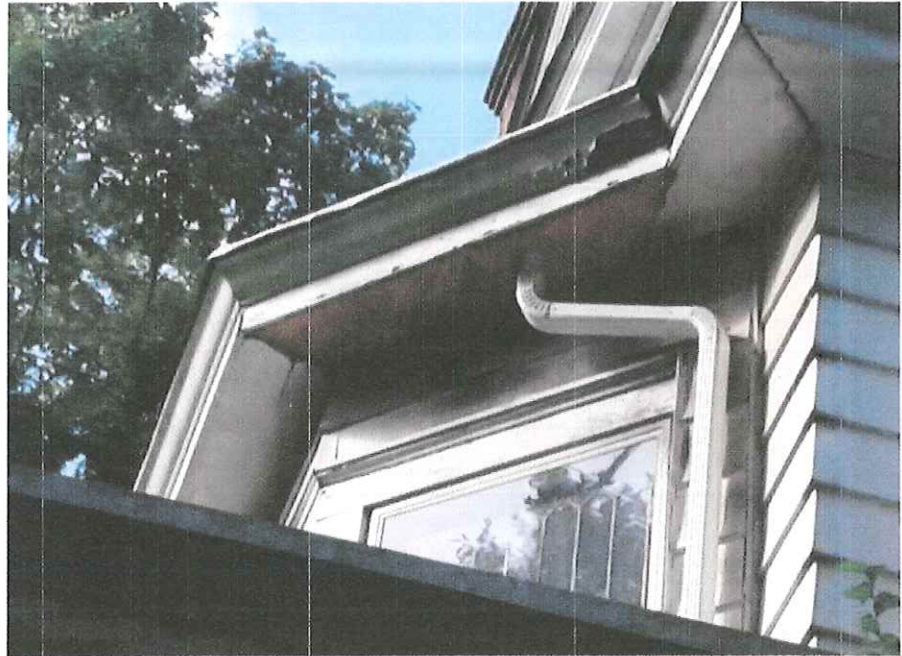
Photograph #13 – Decayed eaves and sills
