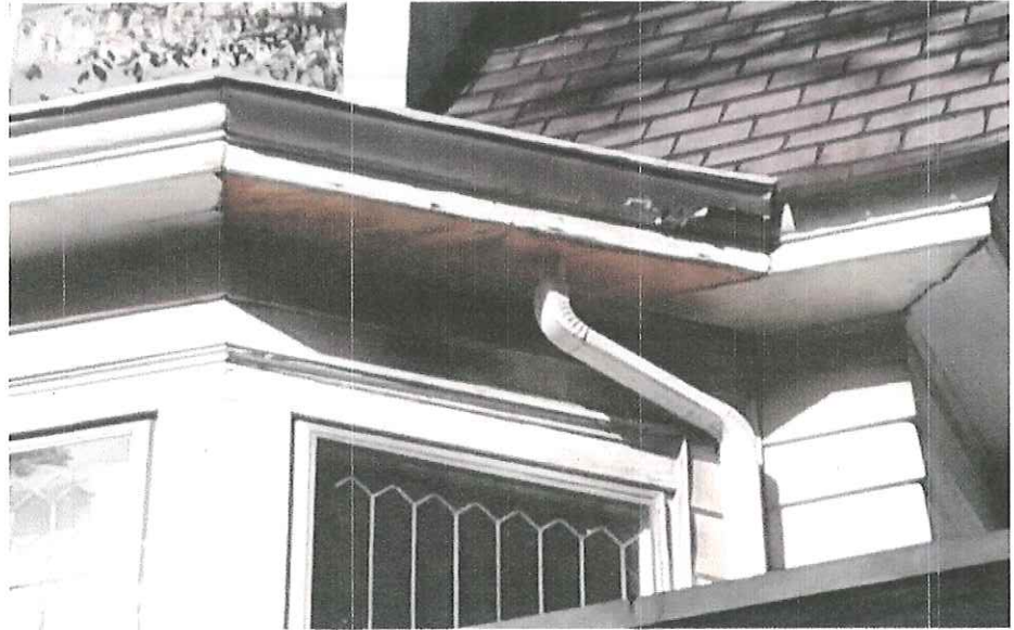
Photograph #15 – Decayed eaves and sills
