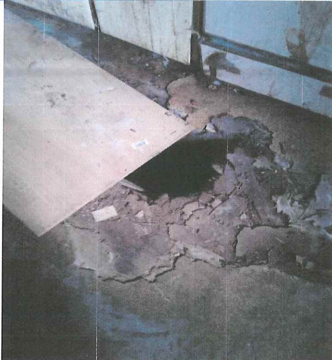
Photograph #9 – Missing floor framing – kitchen
