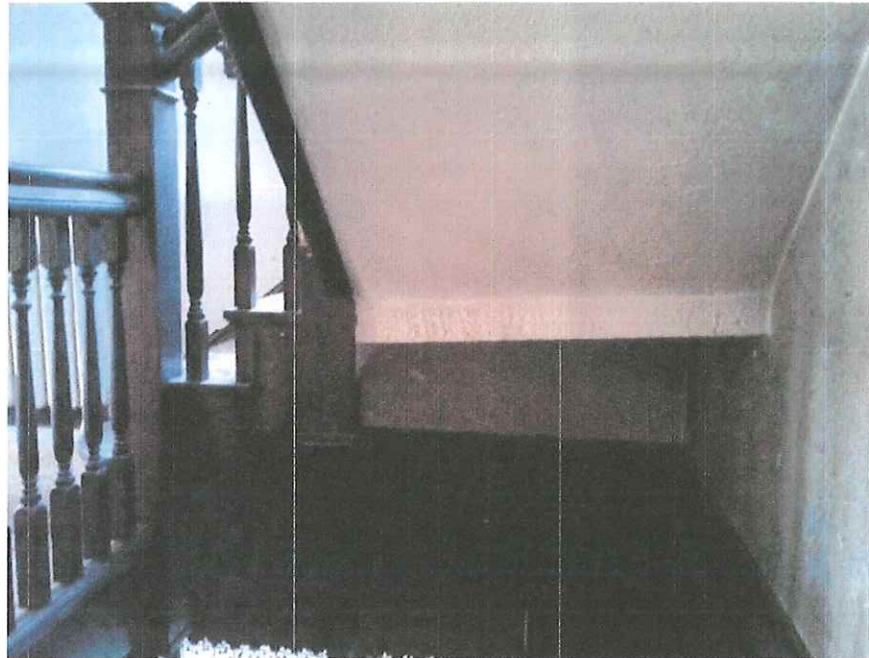
Photograph #11 – Stair deflection and settlement
