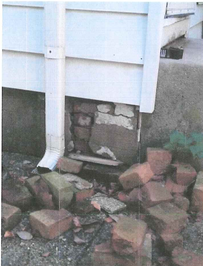
Photograph #10 – Distressed foundation
