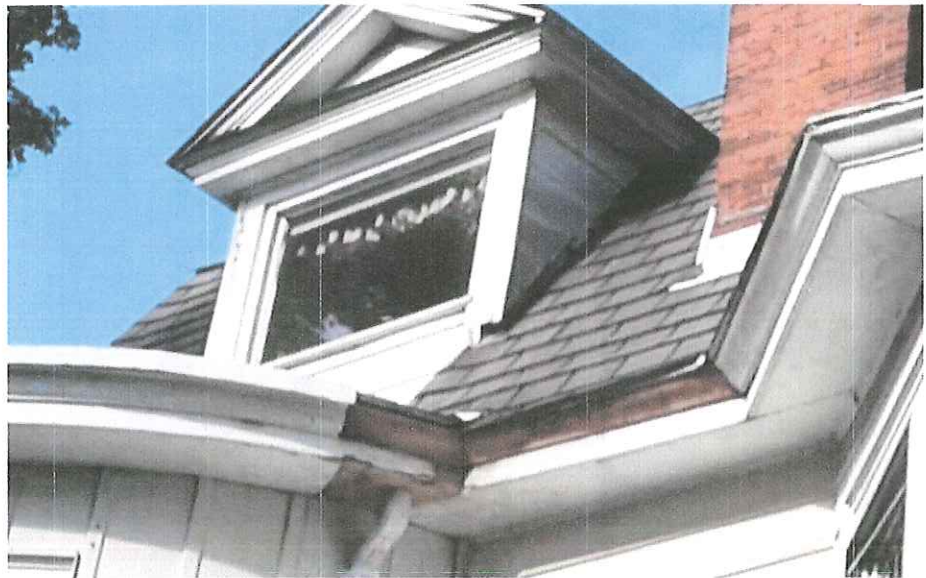
Photograph #14 – Decayed eaves and sills
